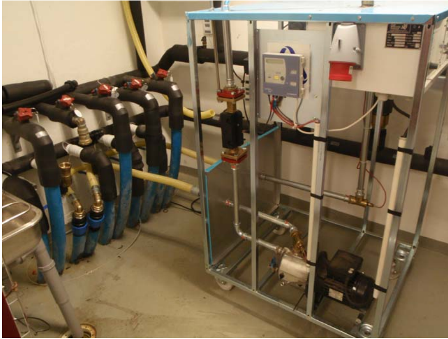
Fig. 2. Used thermal response test equipment.
